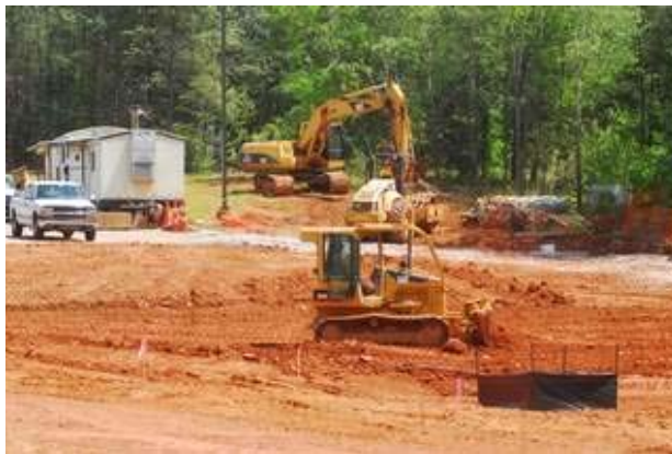
Site work continues at the Clemson University Advanced Materials Center. (JOHN C. STEVENSON/Staff)
